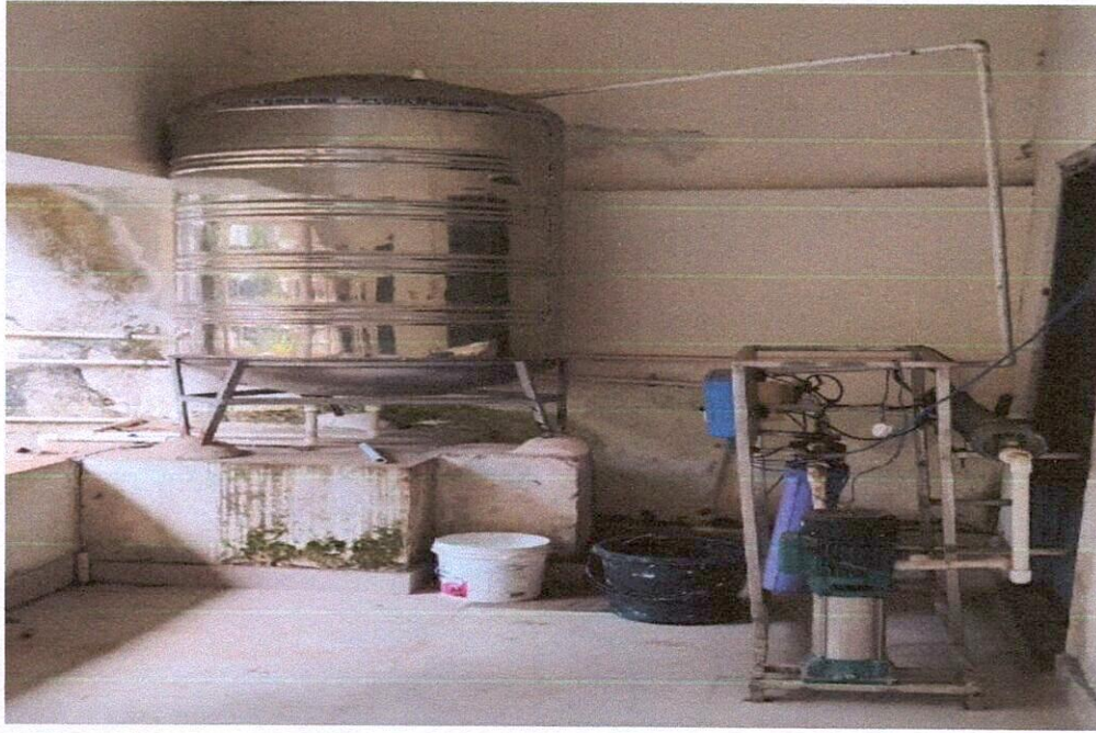
Mineral water plant
